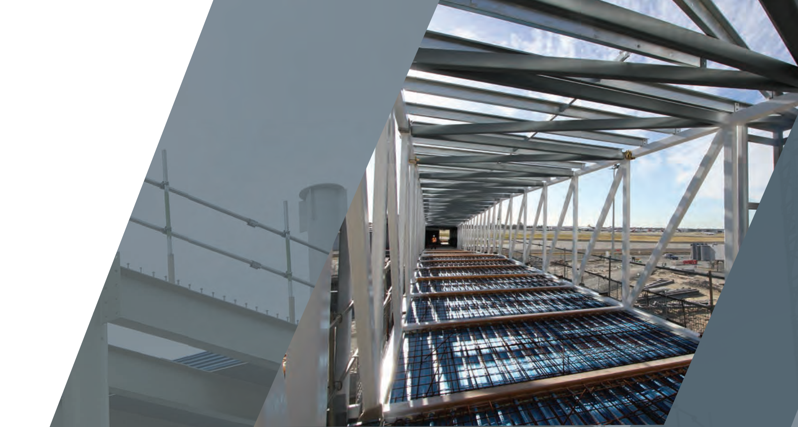
PHOTO: Civmec carried out the fabrication and assembly of approximately 2,500T of painted and galvanised steelwork for the Perth Airport Extension.
