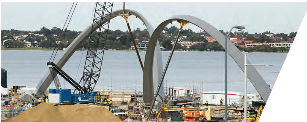
PHOTO: The fabricated pedestrian bridge arches being lifted into place on the Elizabeth Quay Project.
