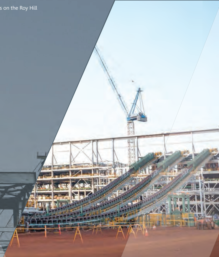
PHOTO: Civmec fabricated and installed 6,500T of structural, platework, conveyor trusses and approximately 30km of process pipework for the Yandicoogina Sustaining Project.
